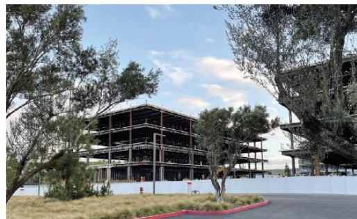
3rd phase of Spectrum Terrace underway, among largest speculative office developments in region
